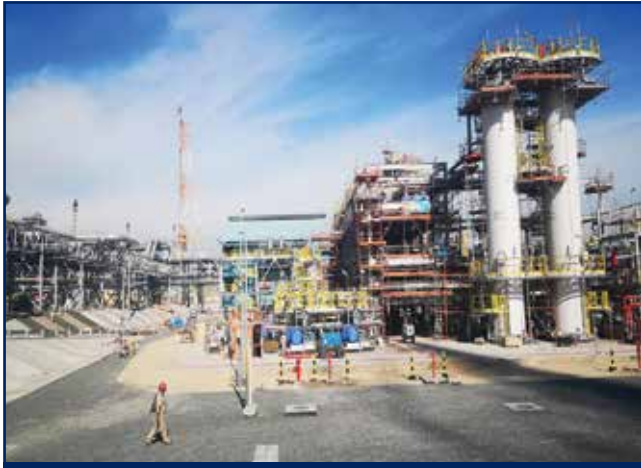
Structural, Mechanical, Piping, Electrical and Instrumentation Works for Sulphur Area at Az-Zour Refinery project - EPC Package 2&3
