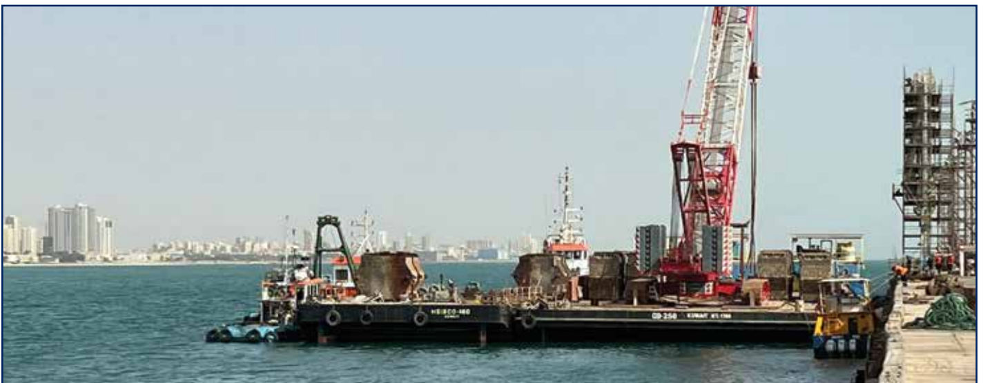
Heavy Equipment Barge for Marine Maintenance Works at Mina Al Ahmadi Refinery
