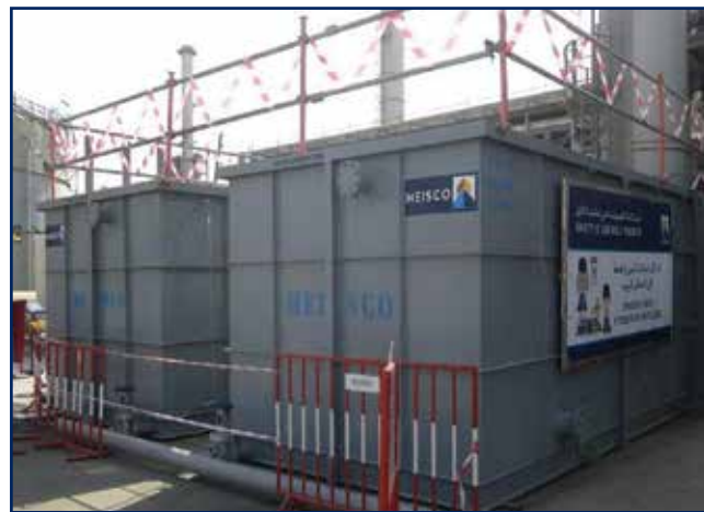
Operations and Maintenance of Bulk Chemicals Facilities, Operational Laboratories and Effluent Water Disposal Plants
