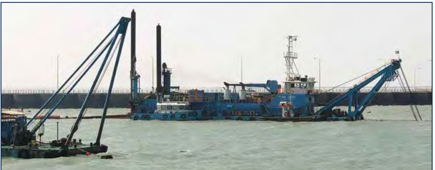
Maintenance Dredging of Seawater Intake Channel at Subiya Power & Water Distillation Station
